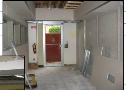
Right - new ramp entrance has an automatic door to help our patrons with strollers and in wheelchairs.
